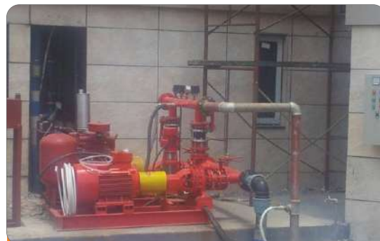
Project: Belanova Apartments Location: Maitama, Abuja. Scope: Fire Fighting Installation
