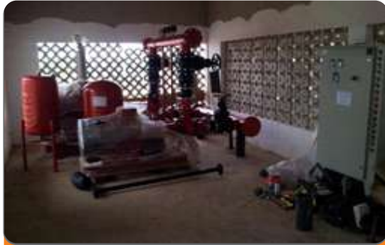
Project: PTDF (School of Petroleum Studies) Location: Kaduna Scope: Installation of 1000GPM Pump (Electro-fusion of HDPE Pipes)
