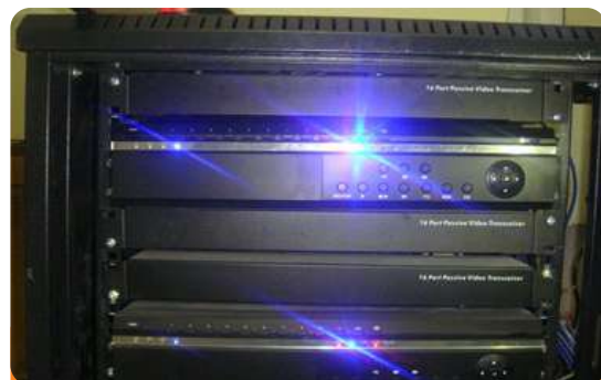
Project: NAF Conference Center Location: Kado District Scope: Fire Detection and Alarm, CCTV, PABX and Public Address System
