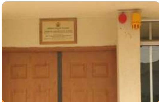
Project: National Institute of Pharmaceutical Research and Development Location: Idu Industrial Layout Scope: Fire Detection and Alarm System
