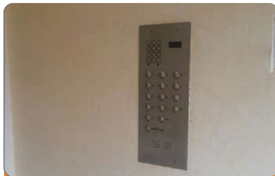
Project: Service Apartments Location: Bourdillion, Ikoyi, Lagos Scope: Fire Detection & Alarm, CCTV, Intruder Alarm PABX, Fire Fighting, Automation, Video Entry System
