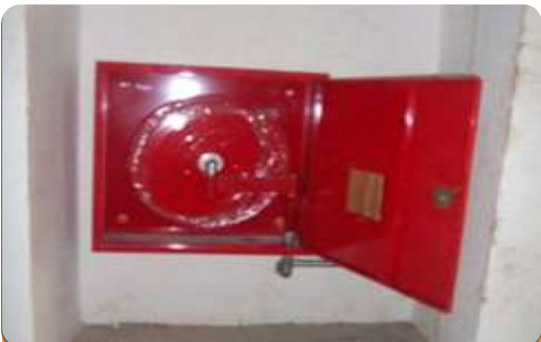
Project: Petroleum Equilization Fund, Headquarter Location: Jabi, Abuja Scope: Detection and Alarm Fire Fighting Installation, Hydrant Installations and Fire Extinguisher Installations
