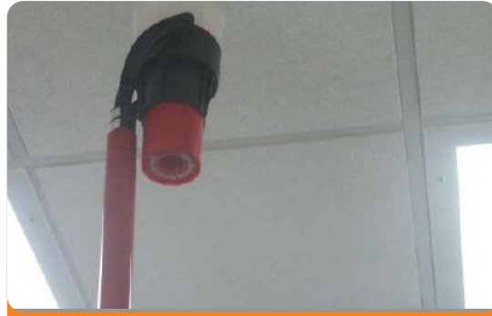
Project: Herdy Crown Nigeria Limited Location: Otedola Jubilee Estate, Lagos. Scope: Fire Detection & Alarm System.
