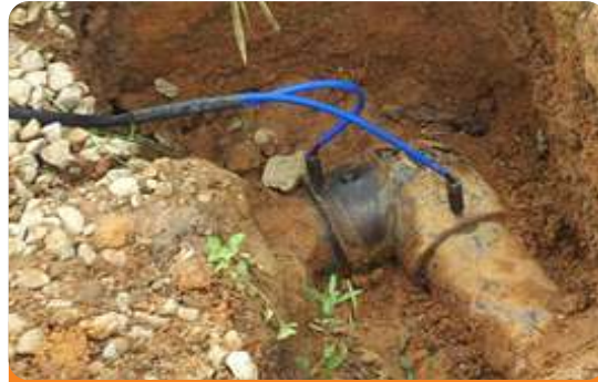
Project: PTDF (School of Petroleum Studies) Location: Kaduna Scope: Installation of 1000GPM Pump (Electro-fusion of HDPE Pipes)
