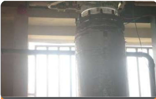
Project: NIPRD (Extraction Plant) Location: Idu Industrial Layout, Abuja Scope: Fire Detection & Alarm System
