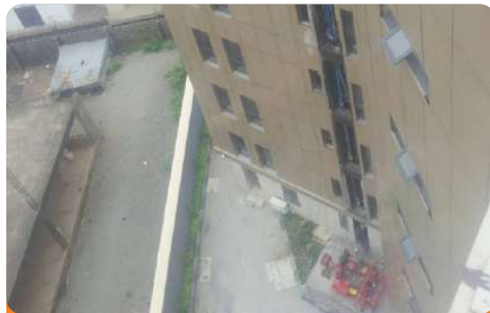
Project: Belanova Apartment Location: Maitama, Abuja. Scope: External Mechanical Services
