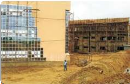
Project: School of Communication Technology, Faculty Building Location: Federal University of Technology Minna Scope: Fire Detection and Alarm, Firefighting and Installations
