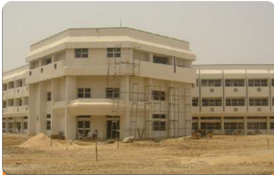
Project: Senate Building Campus, Gidan Kwano Location: Federal University of Technology, Minna Scope: Fire Detection & Alarm, Fire Fighting Installation
