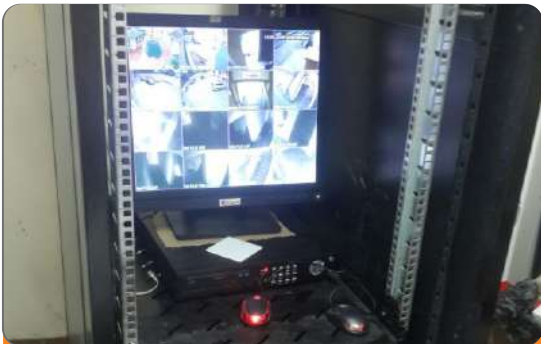
Project: Service Apartments Location: Bourdillion, Ikoyi, Lagos Scope: Fire Detection & Alarm, CCTV, Intruder Alarm PABX, Fire Fighting, Automation
