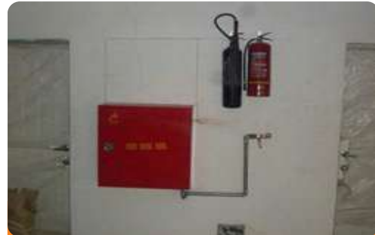
Project: Commercial Office Complex Location: Jabi, Abuja Scope: Detection and Alarm Fire Fighting Installation, Hydrant Installations and Fire Extinguisher Installations
