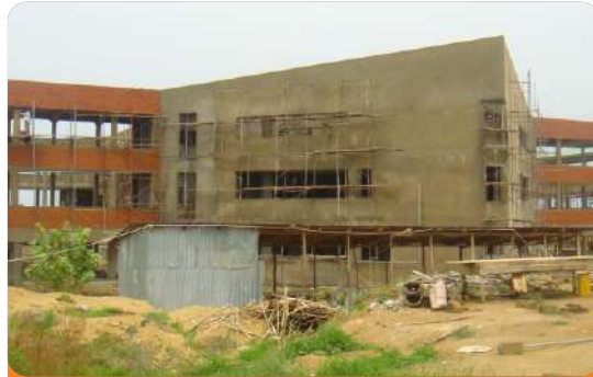
Project: School of Info. & Comm. Technology Location: Federal University of Technology, Minna Scope: Fire Detection & Alarm, Fire Fighting Installation
