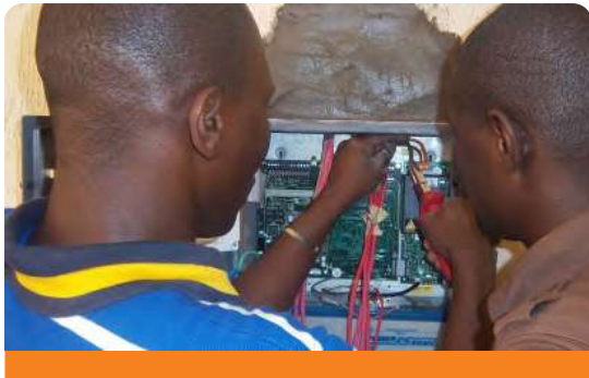
Project: School of Computer Engineering Location: Federal University of Technology, Minna Scope: Fire Detection & Alarm, Fire Fighting Installation
