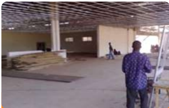
Project: Kitchen and Dining Location: Jos University Teaching Hospital, Jos, Plateau State Scope: Fire Detection and Alarm, Firefighting and Installations
