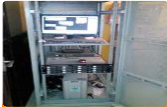
Project: Jabi Luxury Apartment Location: Jabi Luxury Apartment, Kado, Abuja. Scope: CCTV Surveillance Installations
