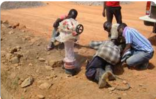
Project: PTDF (School of Petroleum Studies) Location: Kaduna Scope: Installation of 1000GPM Pump
