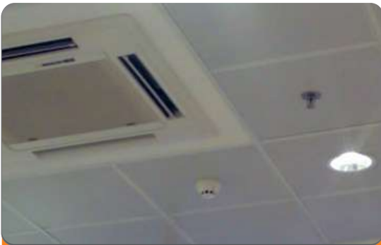
Project: Office Space Location: AF/KLM Office Sheraton Hotel & Towers, Abuja Scope: Fire Detection & Alarm System.
