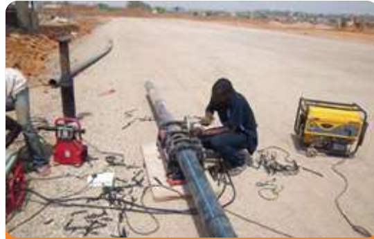
Project: National College of Petroleum Studies Kaduna (NCPSK) Location: KadunaState Scope: Installed Hydrant (Technology Building)
