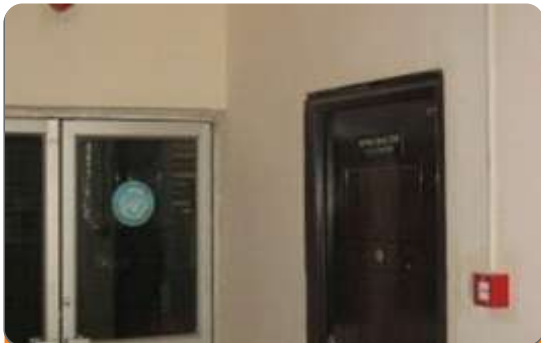
Project: National Institute of Pharmaceutical Research and Development Location: Idu Industrial Layout Scope: Fire Detection and Alarm
