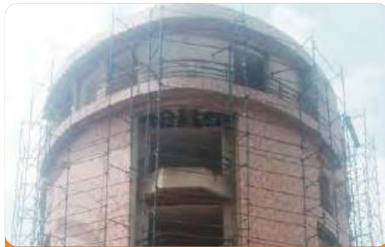
Project: Lilom Engineering Complex Location: Wuse II, Abuja Scope: Fire Fighting Installation
