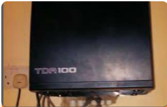
Project: Jabi Luxury Apartment Location: Jabi, Kado, Abuja Scope: Installation of TDA100 PABX Panasonic Console
