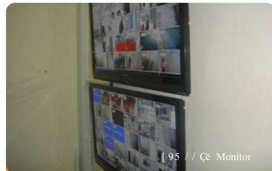
Project: NAF Conference Center Location: Kado District Scope: Fire Detection and Alarm, CCTV, PABX and Public Address System
