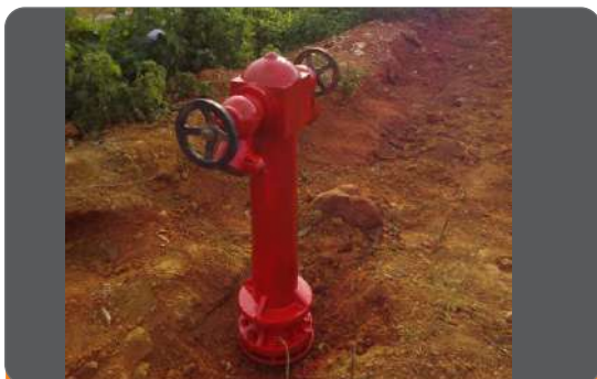
Project: National College of Petroleum Studies (Phase 3 Extension) Location: Kaduna Scope: Extension of 3 Nos Fire Hydrant points using 150mm HDPE Pipes by means of Butt-Fussion and Electro-Fussion Method
