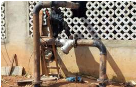
Project: PTDF (School of Petroleum Studies) Location: Kaduna Scope: Installation of 1000GPM Pump
