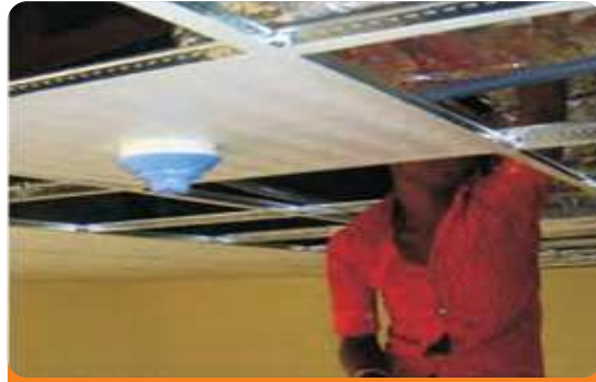
Project: Federal University of Technology Location: Minna, Niger State Scope: Fire Detection and Alarm System.
