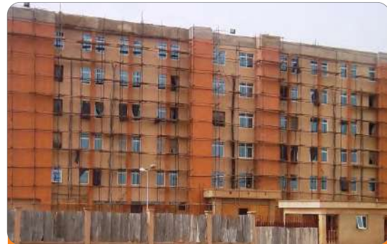
Project: Commercial Complex Location: Jabli, Abuja Scope: Fire Detection & Alarm System, Fire Extinguisher, Fire Fighting Installation, Hydrant Installations
