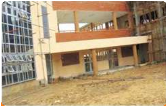
Project: School of Communication Technology, Faculty Building Location: Federal University of Technology Minna Scope: Fire Detection and Alarm, Firefighting and Installations
