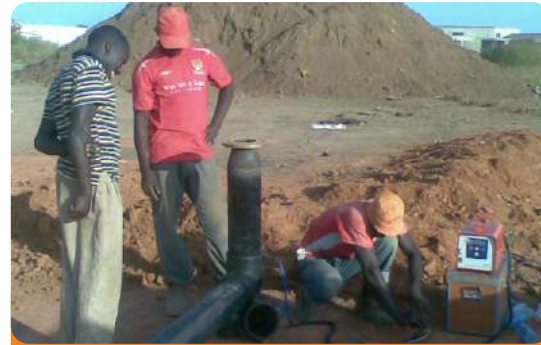
Project: National College of Petroleum Studies Kaduna (NCPSK) Location: Kaduna State Scope: Butt welding of an HDPE Pipes to an Elbow Joint
