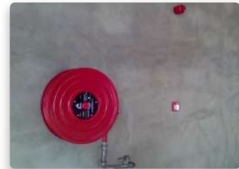
Project: Match Factory Location: Starcase Nig. Ltd. Idu Industrial Estate, Abuja. Scope: Fire Detection and Alarm, Fire Fighting Installations
