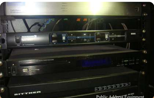
Project: NAF Conference Center Location: Kado District Scope: Fire Detection and Alarm, CCTV, PABX and Public Address System
