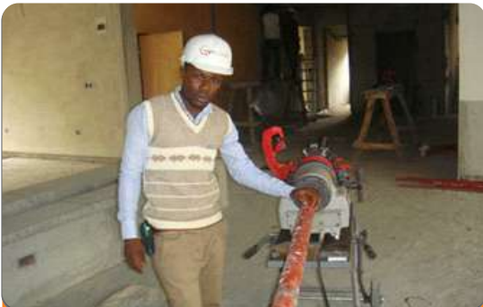
Project: Office Complex, Ryte Cas Location: Wuse II, Abuja. Scope: Fire Detection & Alarm System, Wet Pipe Sprinklers, Wet Riser, Dry Riser & CCTV System
