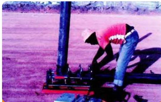
Project: National College of Petroleum Studies (NCPSK) Location: Kaduna Scope: Reducer fixed to HDPE Pipes
