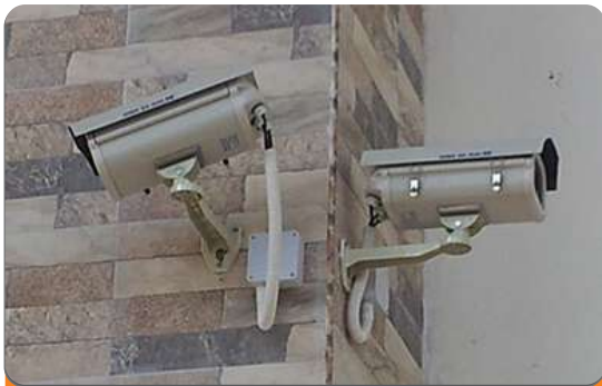
Project: Nigerian Air force Conference Location: Central Area, Abuja Scope: CCTV Surveillance System Installation.
