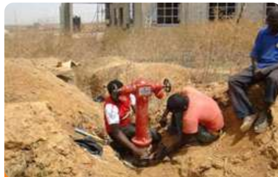
Project: National College of Petroleum Studies Kaduna (NCPSK) Location: Kaduna State Scope: Installed Hydrant (Conference Center)
