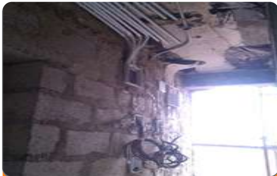
Project: Liberty Suite and Apartment Location: Plot 1806, Cadastral Zone, B13, Guduwa Estate Scope: Firefighting, Wet Pipe Sprinkler, Hose Reel, Fire Hydrant FM200, Dry riser System, PABX, Data and Networking, Hotel Lock, CCTV, PABX and Public Address System
