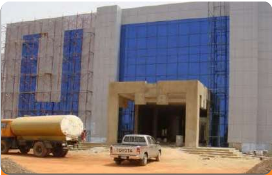
Project: National College of Petroleum Studies (NCPSK) Location: Kaduna Scope: Fire Hydrant Installation
