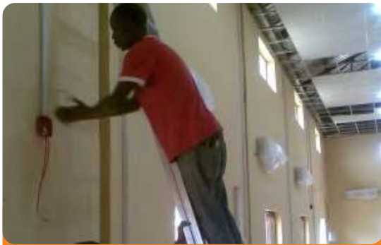
Project: Printing Press Location: Jos, Plateau State Scope: Fire Detection & Alarm System
