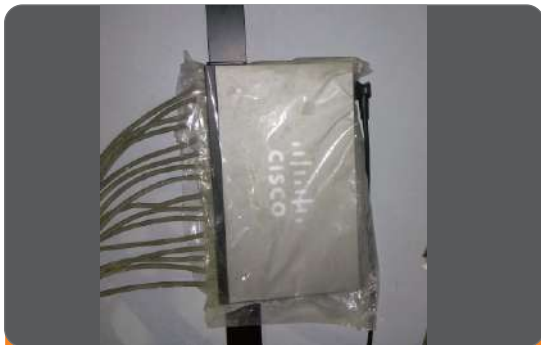
Project: Belanova Apartments Location: Maitama, Abuja. Scope: Data and Networking
