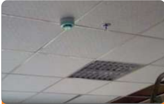
Project: Jeff Bamiro Office Complex Location: Wuse II, Abuja. Scope: Fire Detection and Alarm, Firefighting and Installations
