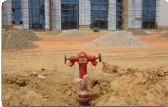
Project: National College of Petroleum Studies Kaduna (NCPSK) Location: KadunaState Scope: Installed Hydrant (Technology Building)
