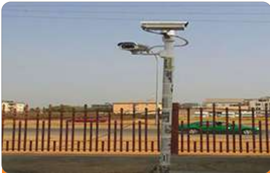
Project: Nigeria Air Force Conference Center Location: Kado District, Abuja Scope: Fire Detection & Alarm System, PABX, CCTV and Surveillance, Public Address System
