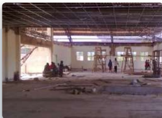
Project: Kitchen and Dinning Location: Jos University Teaching Hospital, Jos. Scope: Fire Detection and Alarm, Fire Fighting Installations
