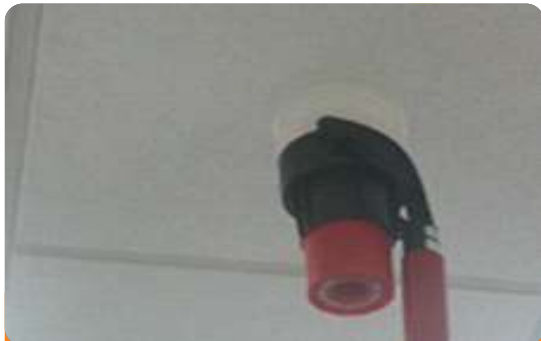
Project: Herdy Crown Nig. Ltd. Location: Otedola Jubilee Estate, Lagos Scope: Fire Detection and Alarm System (Commissioning Process)
