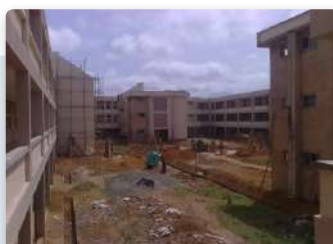
Project: Wards Location: Jos University Teaching Hospital, Jos. Scope: Fire Detection and Alarm, Fire Fighting Installations
