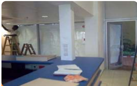
Project: AF/KLM Office Location: Sheraton Hotel & Towers, Abuja Scope: Fire Detection & Alarm
