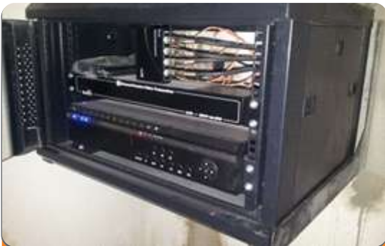
Project: Residential Location: Maitama, Abuja Scope: CCTV, Sprinklers, PABX, Electric Fence.
