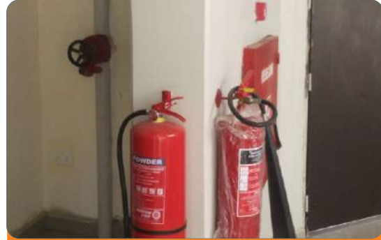
Project: Female Hostel 1 & 2, Block D Location: Federal University of Technology Minna Scope: Fire Detection & Alarm System, Fire Fighting Installation
