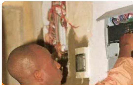
Project: Memorial Hospital Location: New Ederlyey Rd. Calabar, Cross River Scope: Fire Detection & Alarm System
