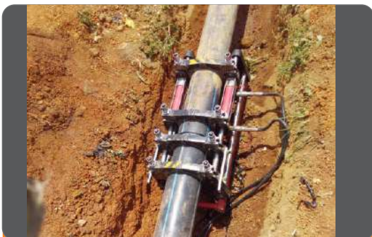
Project: National College of Petroleum Studies (Phase 3 Extension) Location: Kaduna Scope: Extension of 3 Nos Fire Hydrant points using 150mm HDPE Pipes by means of Butt-Fussion and Electro-Fussion Method
